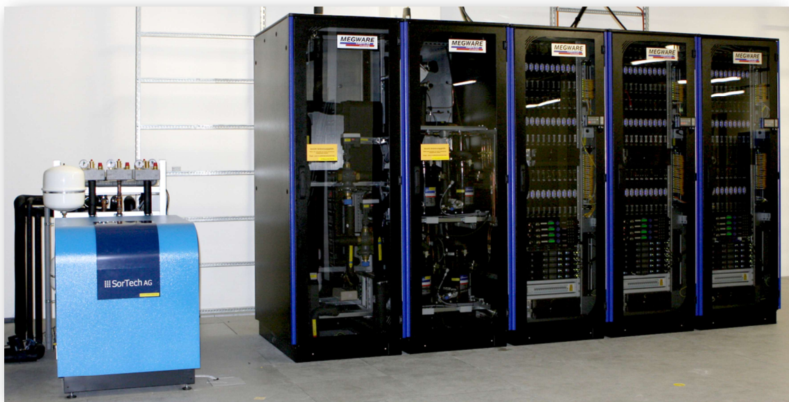
Figure 1: The MEGWARE CoolMUC PRACE-1IP prototype at Leibniz Supercomputing Centre - proof of concept for the re-use of waste heat for heating and chilled water generation.
